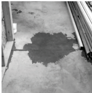
Figure 10.1. Water was leaking into the lower level of Milstein Hall in September 2011, just before it was occupied, in a corridor next to the gallery.
