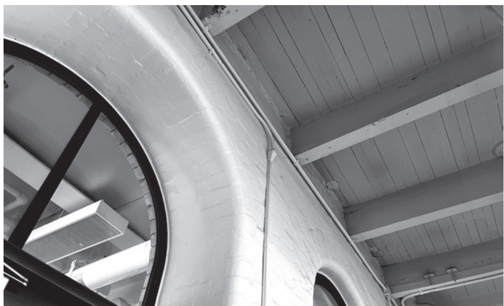
Figure 15.8. Sibley’s brick fire barrier wall is supported laterally by its non-fireproofed wood floor and roof assemblies, shown here at the second floor.
