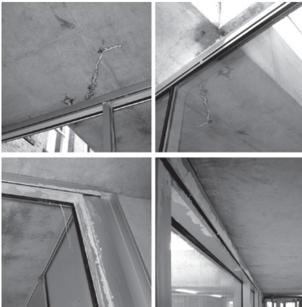
Figure 10.4. Efflorescence in Milstein Hall (July 2013) has occurred where water enters the concrete roof deck, e.g., above the gallery near the loading area, and migrates to interior surfaces, carrying soluble salts.
