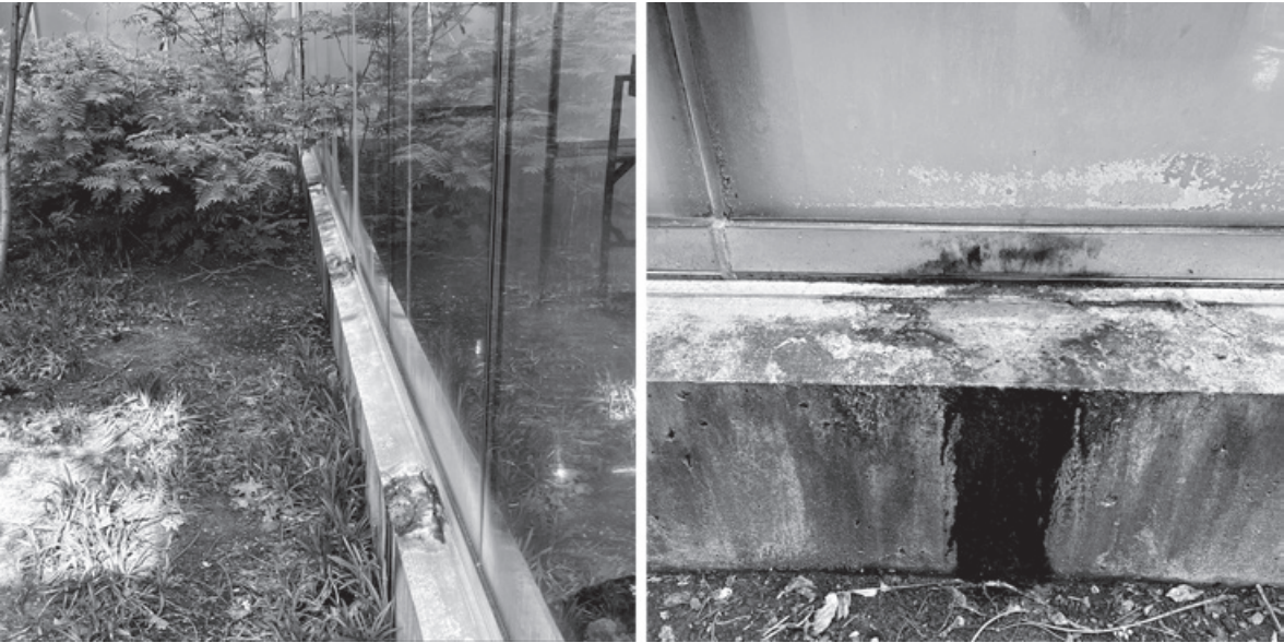
Figure 10.20. Water also picks up some rather nasty artifacts as it enters the concrete, passes through both intended and unintended channels, and drips down to the gallery sill below. (Image taken May 2023.)
