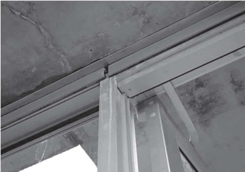
Figure 10.8. Water stains and efflorescence are still visible after a bent metal water stop was inserted into a kerf cut into the concrete ceiling of the Bibliowicz Gallery at Milstein Hall in 2012.
