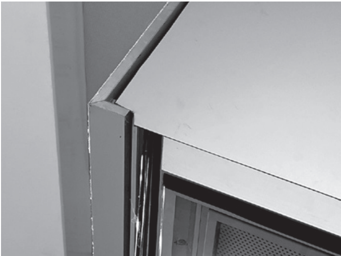
Figure 11.3. Metal panels come together awkwardly at the angled enclosure providing an entrance from second-floor studios to the auditorium below.
