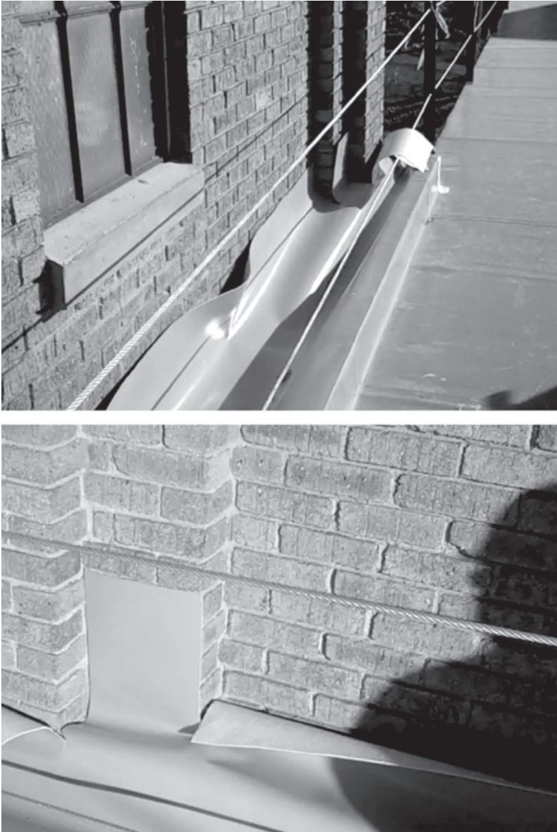
Figure 10.25. The intersection of Milstein Hall's roof with the brick cladding of Rand Hall was sealed with a seismic joint, similar to the joint at Sibley Hall illustrated schematically in Figure 9.6. Here, Milstein Hall's PVC roof membrane is shown prior to the creation of a reglet in the brick wall and the completion of a seismic joint ( top ) and at the challenging geometry where brick protrudes to cover Rand Hall's steel columns ( bottom ).
