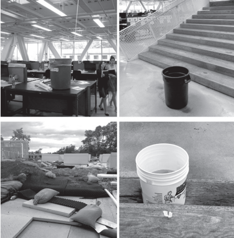
Figure 10.22. Trash cans appeared in Milstein Hall's cantilevered second floor design studios soon after the building was occupied in 2011, placed strategically to catch rainwater leaks from the vegetated roof above ( top left ), both through skylights and at the intersection of Rand Hall and Milstein Hall. Leaks continued in 2015 ( top right ), triggering a major roof repair that lasted for at least two years ( bottom left ), during which time sedums, engineered soil medium, insulation, drainage mats, and protection layers were removed and stockpiled elsewhere on the roof. This major repair also proved unsuccessful, as leaks continued in some of the same places during the fall of 2022—at the stepped auditorium ( bottom right ) and at the intersection of Rand Hall and Milstein Hall (not shown).
