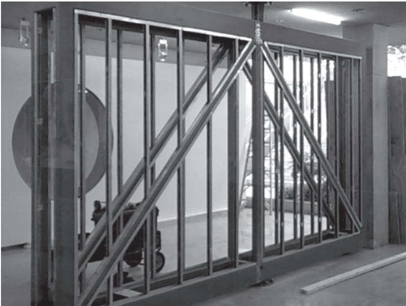
Figure 10.11. The rotating wall in Milstein Hall's Bibliowicz Gallery was taken apart and reconstructed, shown here with the wall finishes removed in the summer of 2012, possibly because of damage caused by excessive deflections in the concrete slab above.
