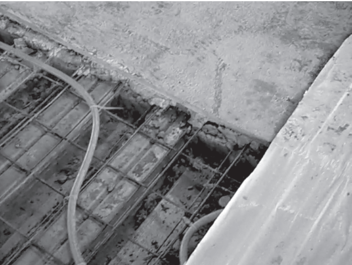
Figure 2.5. Radiant heating tubes are embedded in the structural concrete floor deck of the second-floor studio space.
