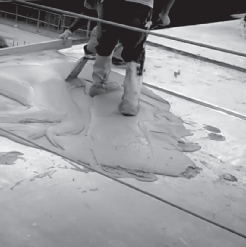
Figure 10.27. Milstein Hall's topping slab is shown being poured over the flat structural slab. The wooden guide for the screed has almost no inclination and certainly not a two-percent slope.
