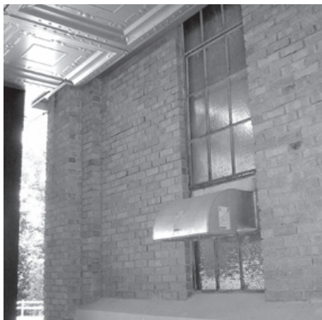
Figure 15.6. Openings in the fire barrier between Milstein and Rand Halls have neither opening protectives nor fire dampers.
