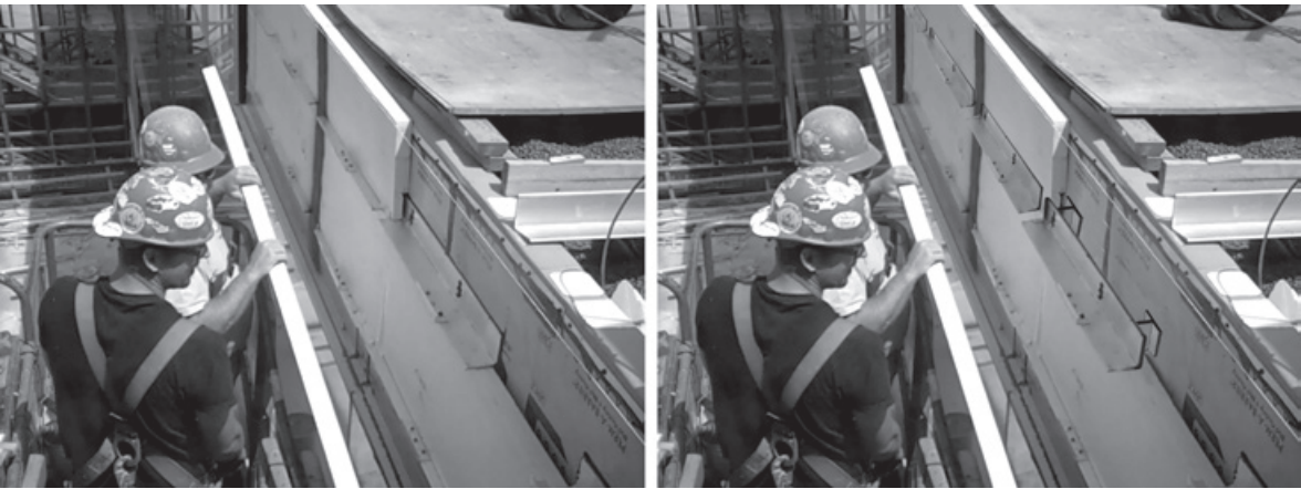
Figure 9.2 A significant thermal bridge can be seen in this construction photo of Milstein Hall ( left ), with horizontal steel angles, to support stone cladding panels, interrupting the thermal control layer, i.e., the rigid insulation. I’ve revised this screen-captured image to illustrate how a “stand-off” works ( right ): the horizontal angle would need to be moved 2 inches (50 mm) away from the sheathing and air barrier so that rigid insulation can be placed behind the steel angle, minimizing the thermal bridging.
