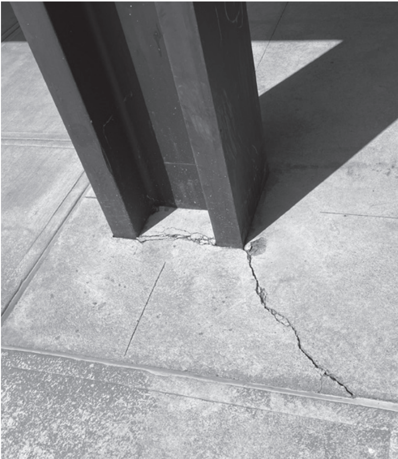
Figure 11.13. With no isolation joints at exterior columns, slab cracking is fairly predictable.
