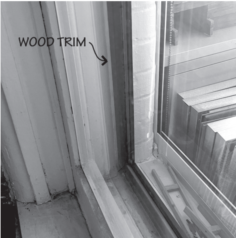
Figure 15.4. Fire-rated glazing is installed directly in front of wood framing for the existing window in the fire barrier wall between Milstein and Sibley Halls.
