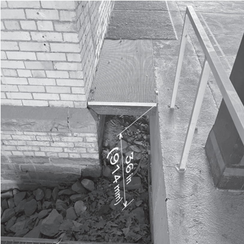
Figure 12.1. Guards are both missing and, where they appear, noncompliant at the grated bridge connecting Milstein Hall’s arcade to Sibley Hall.
