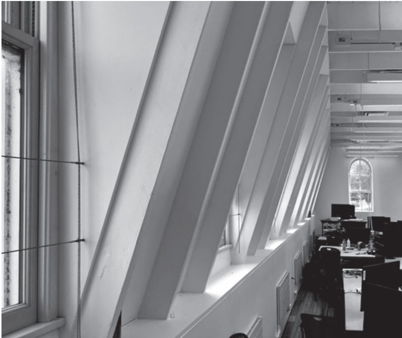
Figure 14.1. The inclined wooden structure of Sibley Hall’s Mansard roof downgrades its construction type from IIIB (fire-rated masonry exterior walls and wood-framed floors and roof) to VB (non-fireproofed wood frame).
