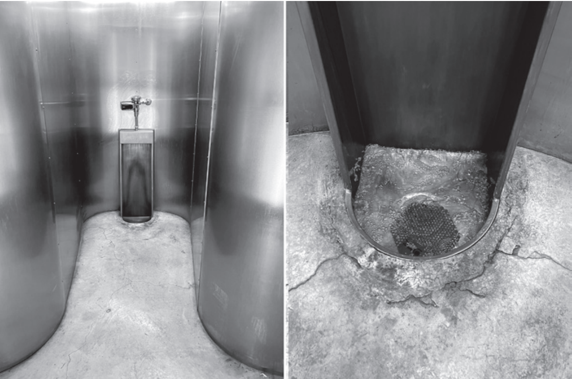
Figure 2.2. Stainless steel urinals in Milstein Hall are built into the noncompliant (cracking) concrete floor slab and cannot easily be repaired or replaced.
