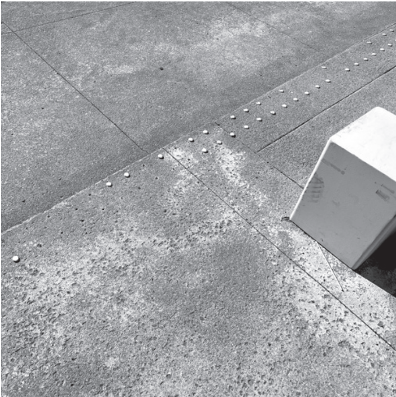
Figure 6.16. The discontinuity of Milstein Hall's plaza and the loading area, even with the addition of tactile circular discs, is extremely hard to pick up, especially in the late afternoon or early evening when there are no shadows cast by the western sun.
