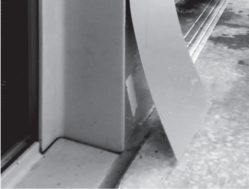
Figure 11.7. Poorly detailed metal cladding has delaminated near the exterior stair exit door on the second floor.
