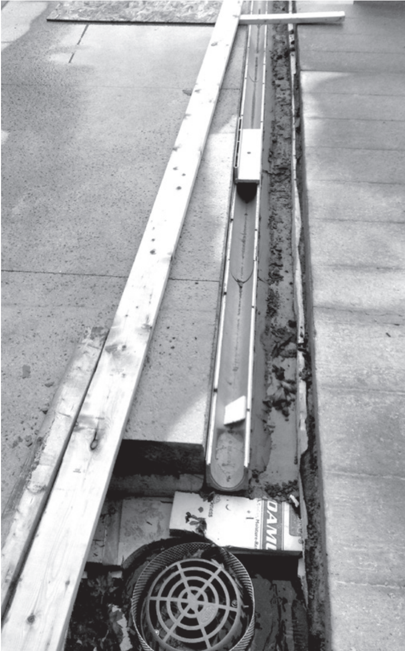
Figure 10.13. The topping slab of Milstein Hall's plaza deck was cut at the approximate low point and most of the rigid insulation was removed to accommodate a linear channel, sloping to a new drain.
