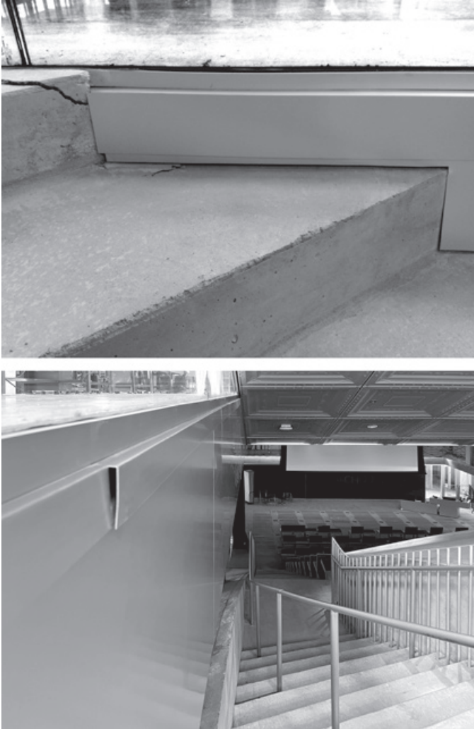
Figure 11.4. Metal trim creates an awkward transition between the Miesian “box” of the second floor and the concrete “blob” that includes auditorium stairs.
