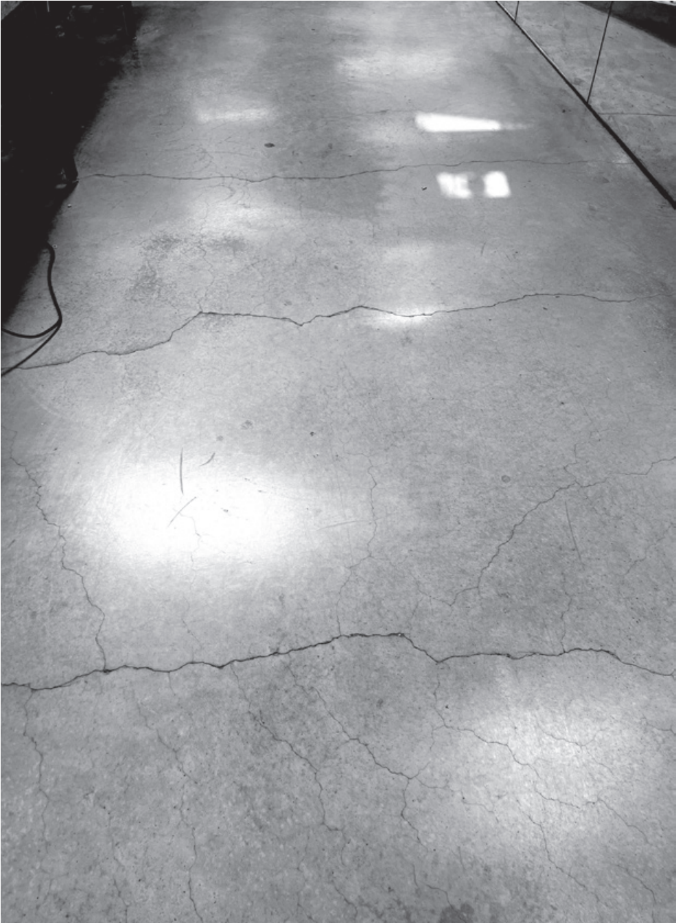
Figure 11.11. Cracks appear not only at re-entrant corners of Milstein Hall's second-floor slab, but also throughout the general field.
