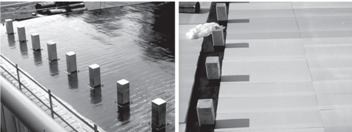
Figure 9.3. Bollards are installed directly on the structural concrete slab above occupied and heated space ( left ); insulation boards are then placed around the bollards ( right ).
