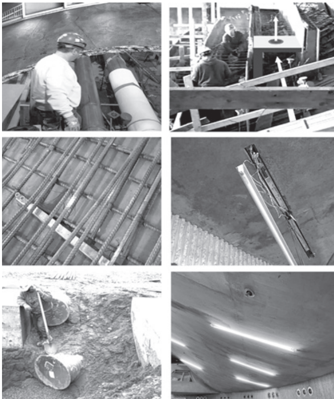
Figure 2.6. Mechanical, electrical, and fire safety items buried within structure: storm drainpipes within concrete dome ( top left ); conditioned air plenum within concrete seating structure in auditorium ( top right ); lighting fixture cut-outs in the Crit Room dome placed in formwork ( middle left ); cutout in dome concrete, ( middle right ); mechanical ducts below slab-on-ground ( bottom left ); and sprinkler pipes embedded in concrete ceiling above Crit Room and elsewhere ( bottom right ).
