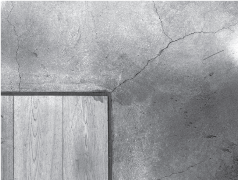
Figure 11.10. Cracks have proliferated throughout the topping slab on the second floor of Milstein Hall; especially at corners—here, where the wood floor area meets the concrete.
