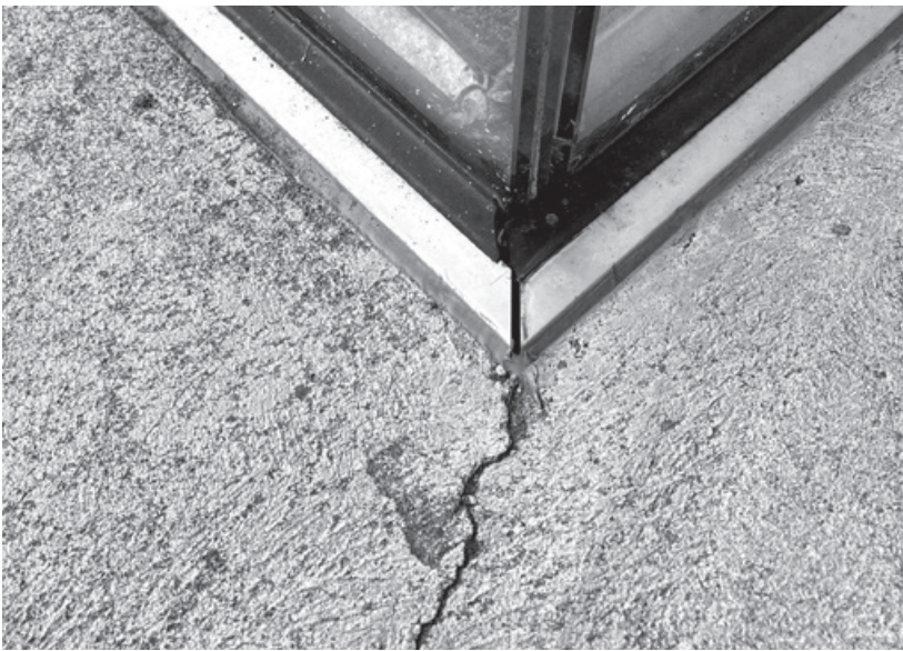
Figure 10.18. Water can enter the concrete slab of the plaza deck through cracks in the concrete and openings in the glass guard inserts around the sunken garden, above the below-grade gallery. (Image taken May 2023.)
