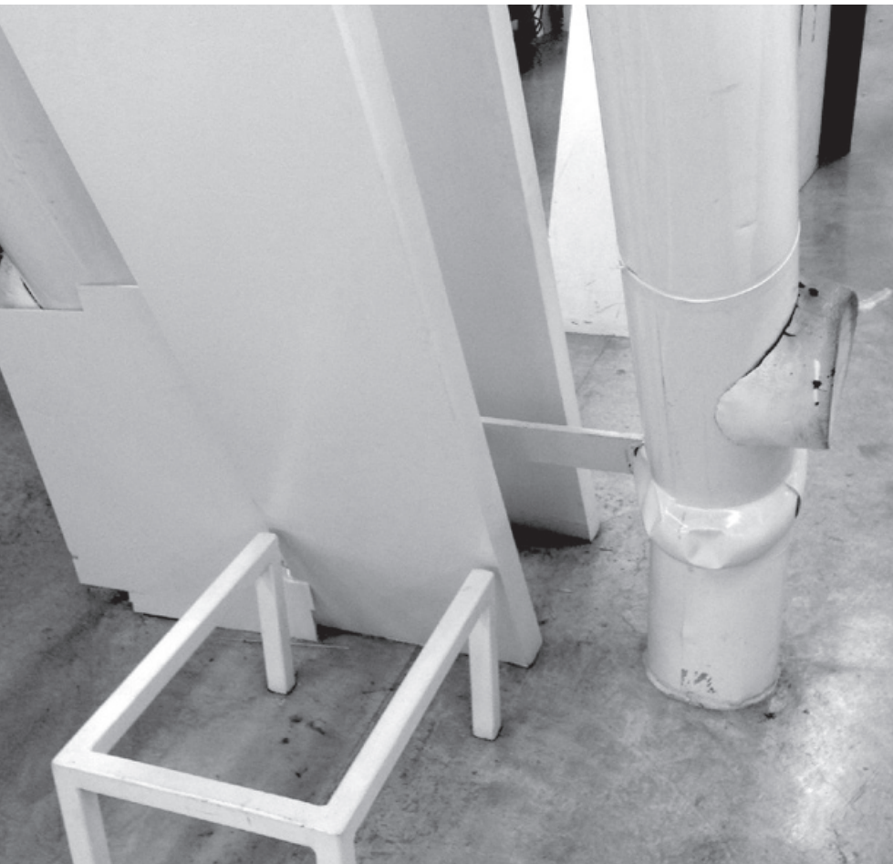
Figure 20.8. Milstein Hall’s rainwater system originates in drains on the vegetated roof, courses through several large drainpipes, shown here in the second-floor studios, continues through the outer layers of the Crit Room dome (as shown in figure 2.6), connects into the regional storm sewer system under University Avenue, and finally is discharged, untreated, into Cayuga Lake.
