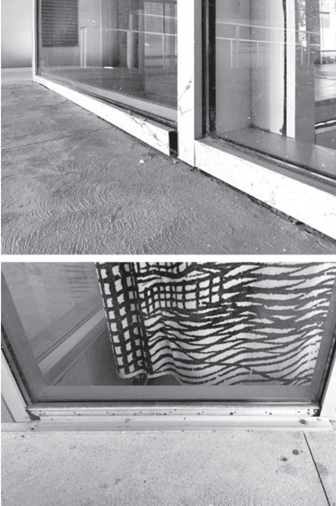
Figure 11.6. Curtain wall sill cover plates have partially or completely detached at the north side of Milstein Hall's lobby ( top ) and at the west side of the auditorium ( bottom ).
