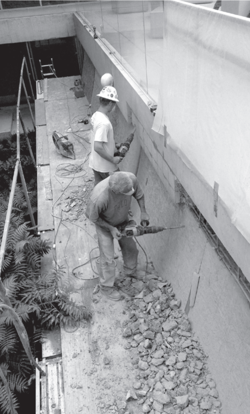
Figure 10.15. Workers remove most of the concrete fascia of Milstein Hall's Bibliowicz Gallery.
