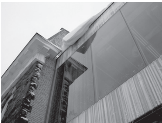
Figure 12.5. Hunks of snow often cantilever out over the roof edge of Milstein Hall, which has no protective parapet or railing.
