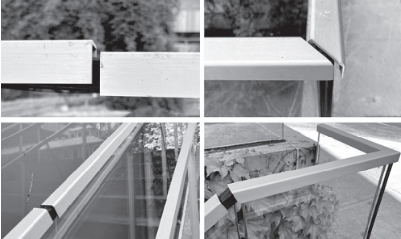
Figure 11.8. Aluminum trim pieces at the top edge of exterior glass guards are coming apart at their joints.
