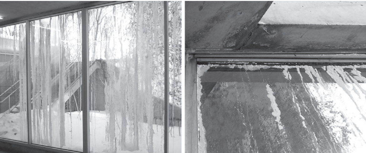
Figure 10.9. The Bibliowicz Gallery windows at Milstein Hall were covered in efflorescence due to water leaking through the plaza deck above (March 2015).
