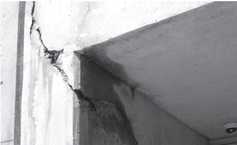
Figure 11.17. A large crack appeared in Milstein Hall’s basement-foundation wall immediately adjacent to the concrete retaining wall to its left, shown here in 2013.
