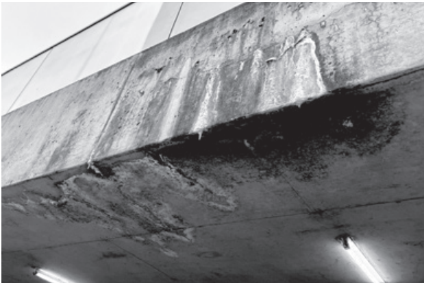
Figure 10.5. Efflorescence can still be seen on the soffit and fascia of the concrete deck supporting the loading area at Milstein Hall, more than a decade after its construction (image taken May 2023). Stalactites, possibly caused by dissolved cement stone, are an indication of a potential structural problem.
