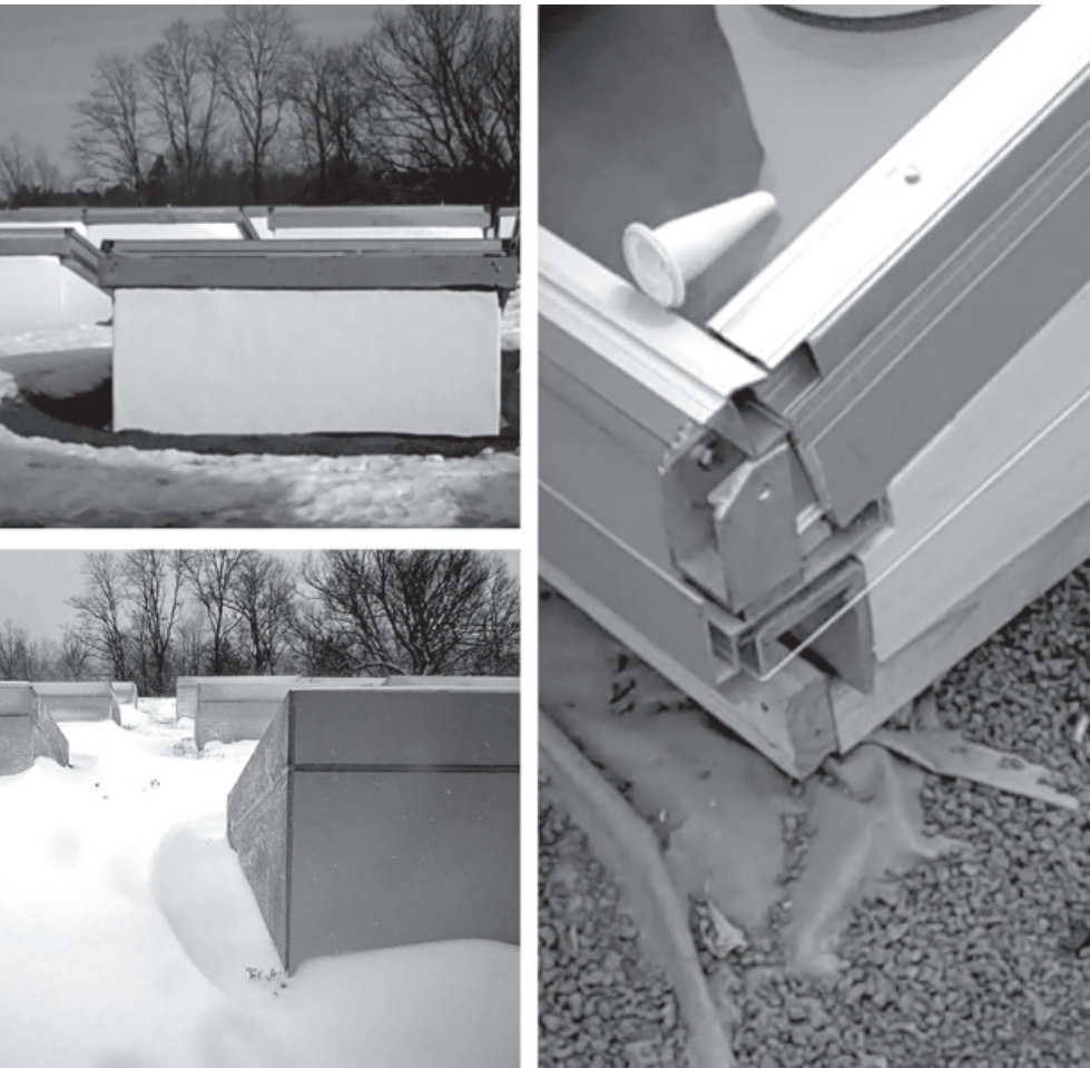
Figure 9.9. Effects of heat loss can be seen in circles of melted snow around uninsulated skylights during construction ( top left ); insulation adhered to concrete skylight curbs is not continuous with horizontal insulation placed over the roof deck, creating thermal bridges ( right ); and because the reinforced concrete skylight insulation is not continuous, the effects of heat loss (thermal bridging) can be seen in the adjacent depressions within the otherwise even bed of snow ( bottom left ).
