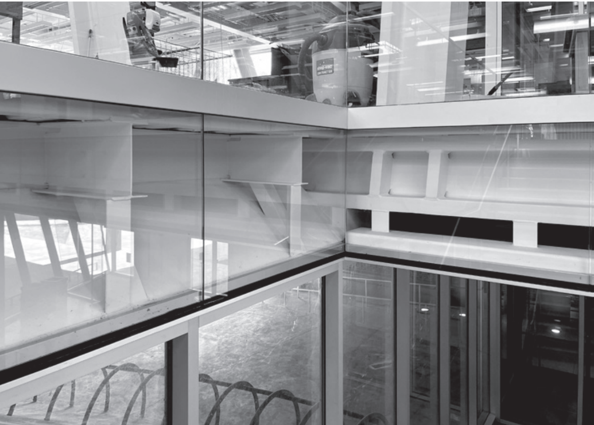
Figure 11.1. Glass panels at the second-floor stair opening create what amounts to a structural display case.
