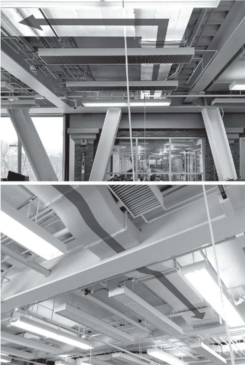
Figure 2.4. A duct for outside air distribution—labeled “A” in figure 2.3—is shown emerging from adjacent Rand Hall, where the mechanical room is located one level above ( top ). These ducts carrying fresh air are threaded through the webs of structural steel beams ( bottom ), making future alterations difficult. Light fixtures and matching chilled beams can be seen just below the ducts. Illustrative arrows added by the author.
