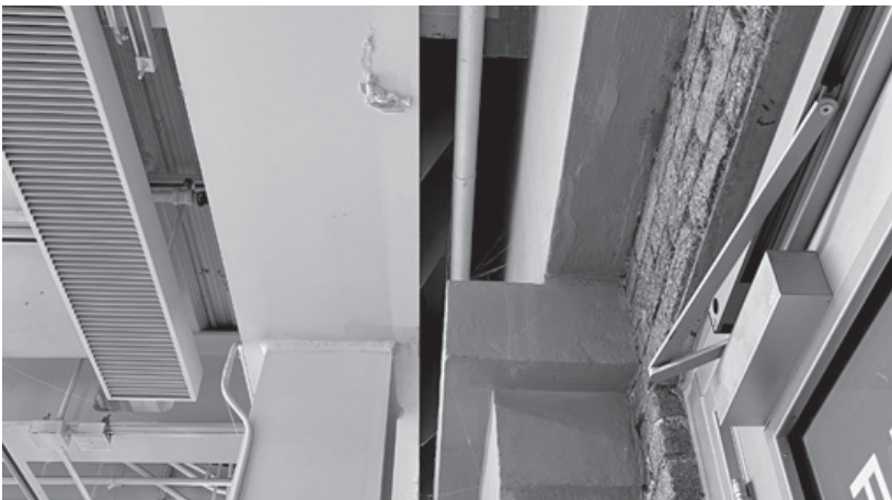
Figure 9.8. Seismic joints between Milstein Hall and Rand Hall create a 5-inch (127 mm) uninsulated gap where the buildings come together.
