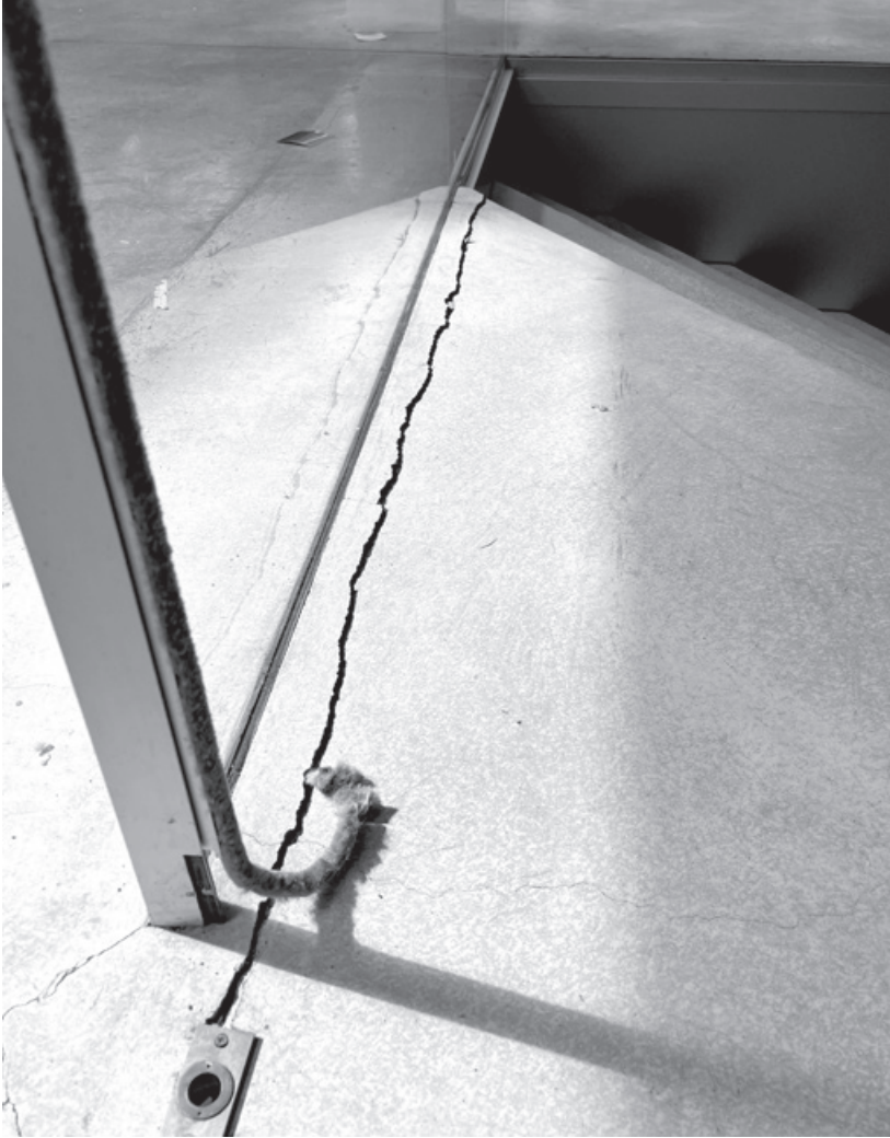
Figure 11.5. Major concrete slab cracking has occurred at the second-floor entrance to the Milstein Hall auditorium; the acoustic seal for the sliding door is also falling apart.
