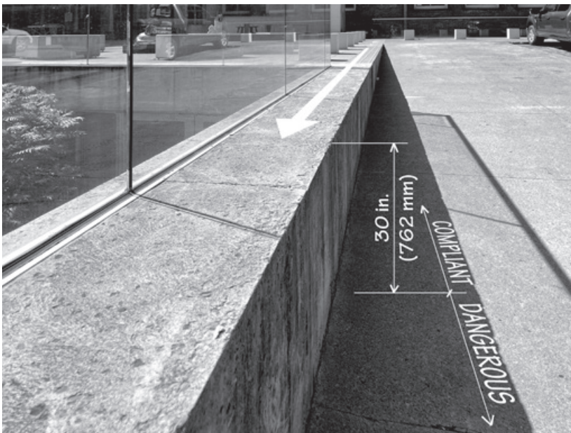
Figure 12.2. The flat plaza concrete deck transitions seamlessly into the top surface of a concrete wall separating the loading area from the sunken garden, creating a vertical discontinuity with no guard rail.
