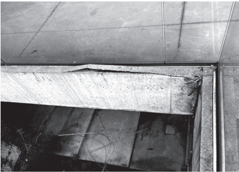
Figure 10.19. Even after substantial renovation of the gallery fascia and plaza deck in 2015, major spalling of concrete is occurring at the fascia-deck intersection. (Image taken July 2023.)
