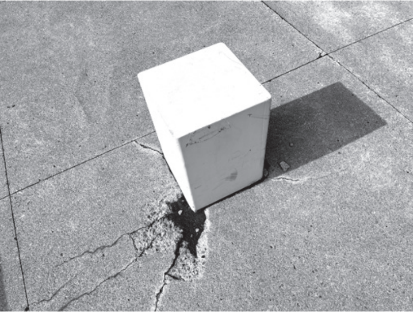
Figure 9.4. Concrete cracking and slight displacement of the bollard suggests a vehicle-bollard collision that may have compromised the waterproofing hidden below grade.
